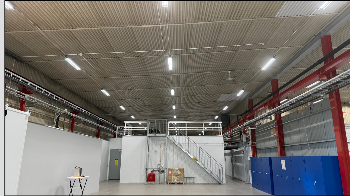
LED lights in general areas
